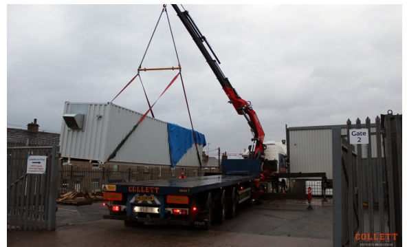
Collection of the mobile plant room for delivery. At the PPS head office in Brighouse
