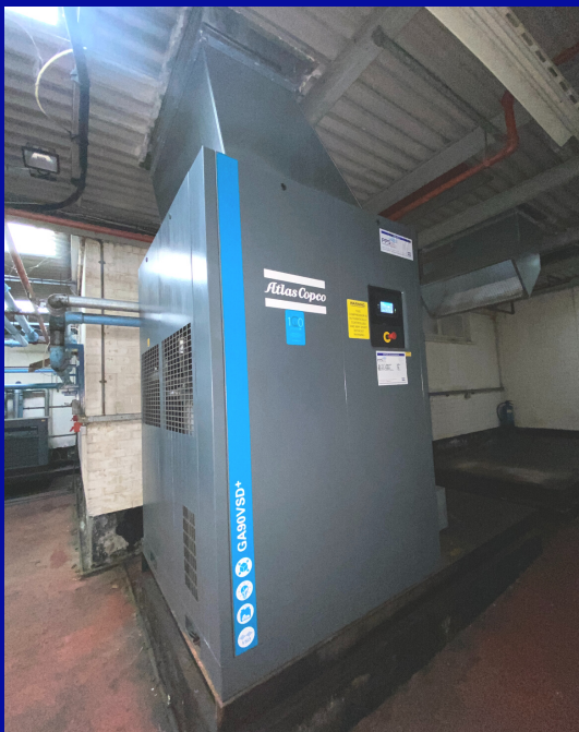
Newest, energy efficient unit
